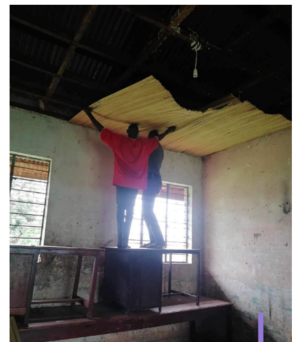
Samson and Ronald putting up a ceiling to make a student common room out of a store room.
